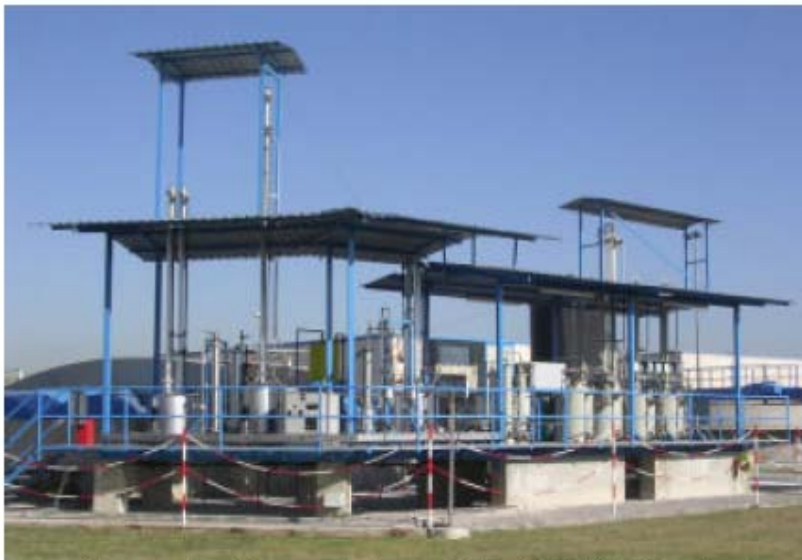
Figure 1 – General view of the BioEDAR plant
